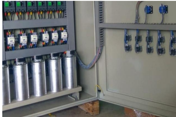
Figure 1. Capacitor Bank (sources: galleoncy)
